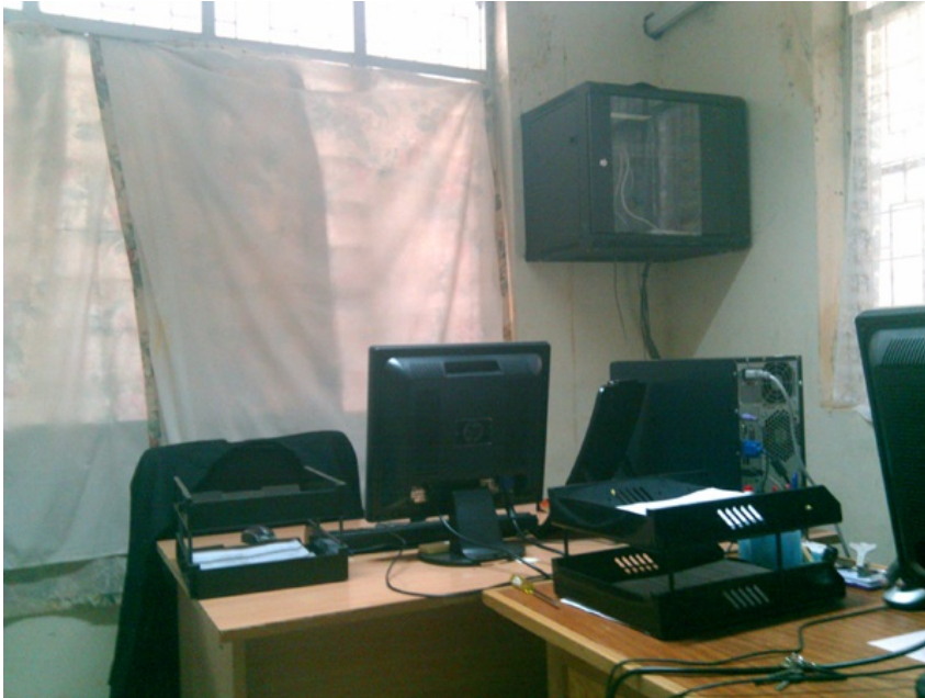
OpenMRS server room in Webuye, Kenya.
